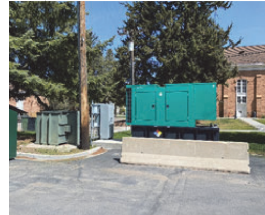
Generator and ATS
