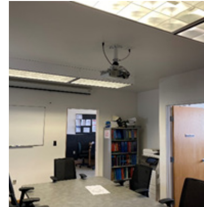
T8 Troffers and older technology systems can be seen in the image above.
