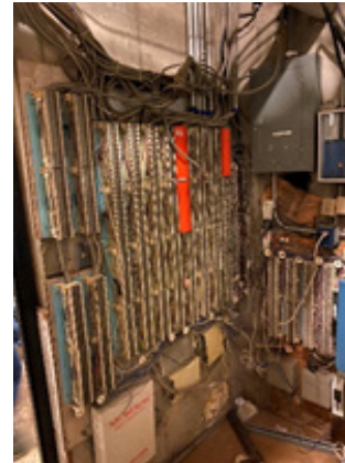
Telecom service blocks
