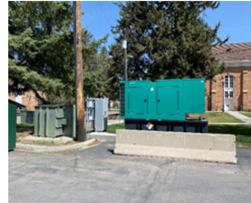
Generator and ATS
