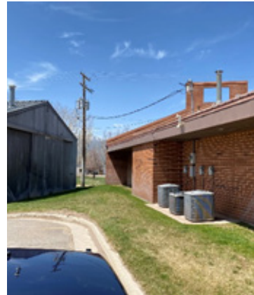
Overhead utility transformer connection at the rear of the building.
