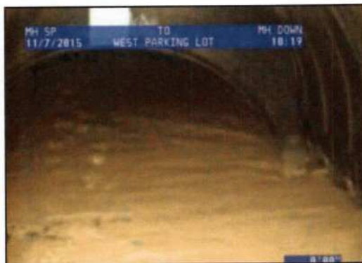
SEPARATOR ROW: Separator Row prior to cleaning
