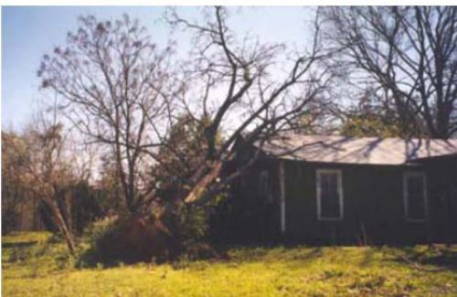
Figure 5: The weight of this tree could cause this part of the home to fall
