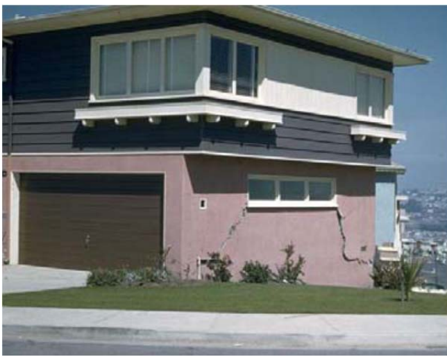
Figure 1: Cracks in a masonry are a sign of danger.
