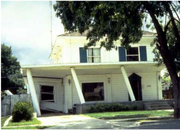
Figure 3: Leaning porch after an earthquake
