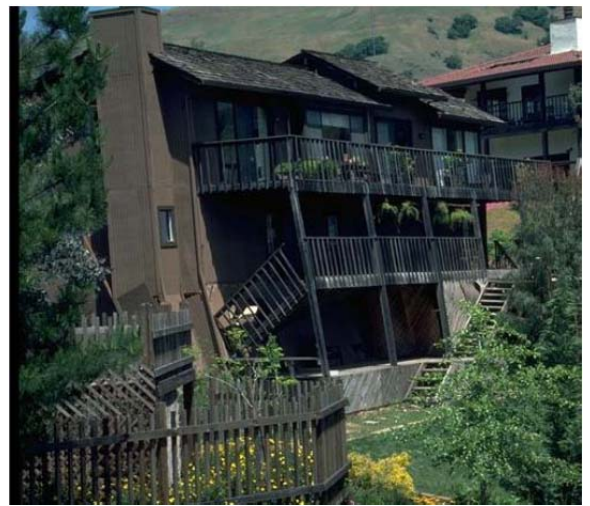
Figure 2: Notice the entire wall near the chimney is out of plumb.
