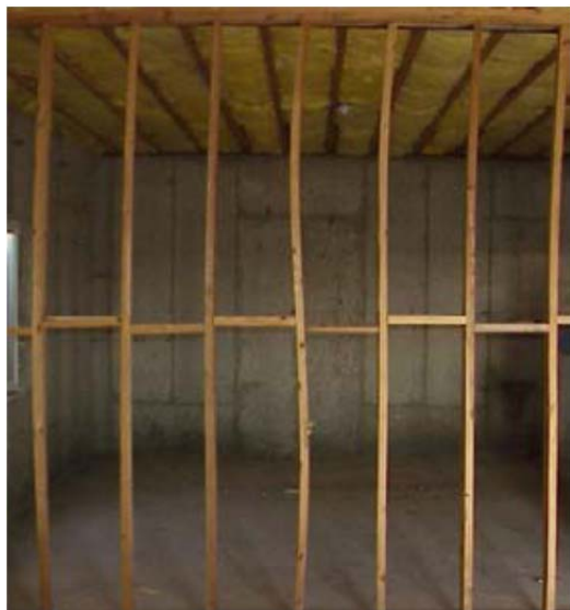
Figure 7: Notice the middle stud is deformed in an "S" shape.
